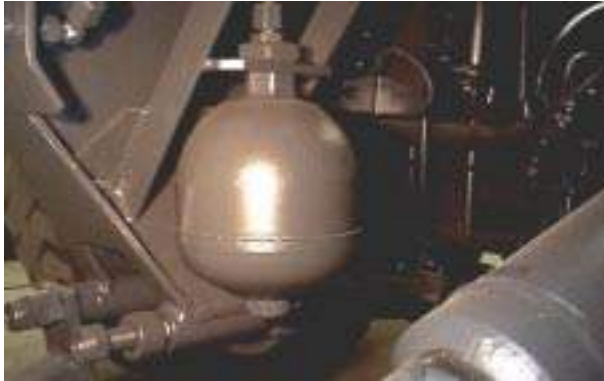
Emergency steering accumulator
