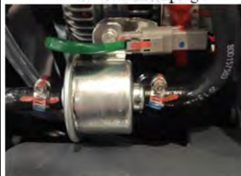
Fuel supply pump.
