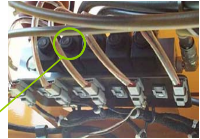
-Location: Main pump room -Spec: 24V, 15~25Ω
