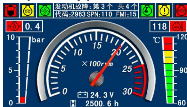
Figure 2 Home page----alarm condition
