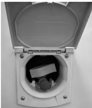
External gas socket
