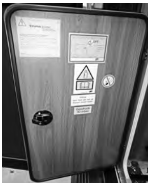
Safety instructions in gas bottle container
