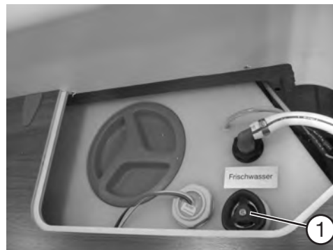
Outlet valve for fresh water tank
