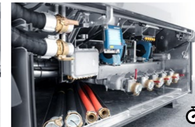
8 Direct discharge lines
